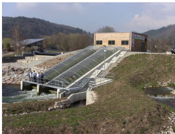
Fig-2 Two Parallel Screw Turbines (2x250 kW)
