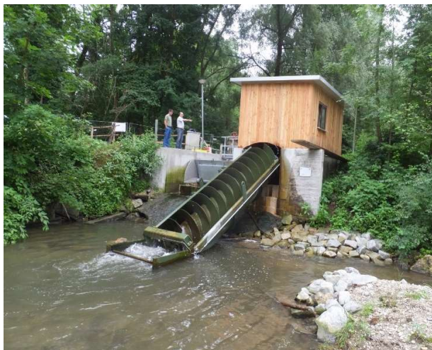
Fig-3 Installed Archimedean Screw Turbine
